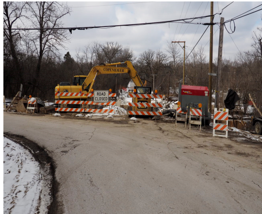
Bridge closed at Cuba/Merry Oaks Road
